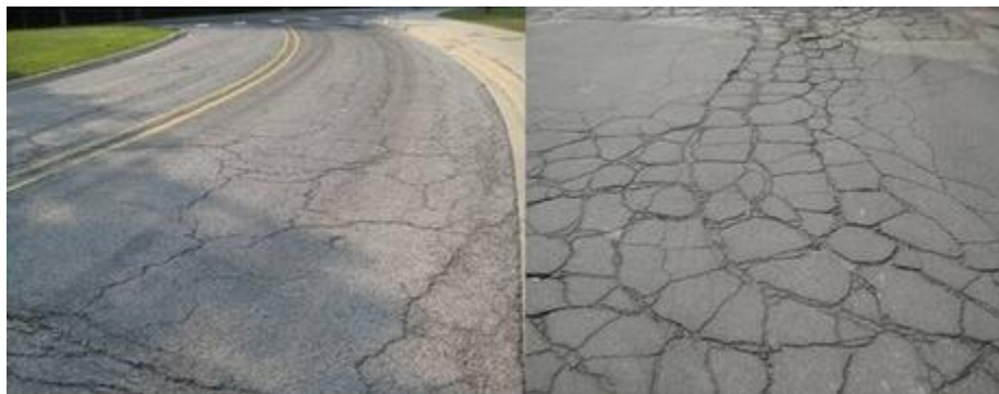
Figure1: Raveling /Rutting (Park, P.,n.d)
