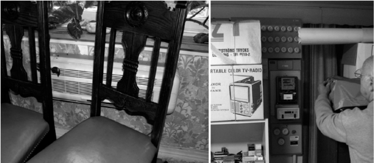
Figure 2: Left, an air pump hidden behind chairs. Right, an informant uncovering an electricity meter in the basement.
