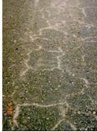
Figure 1.2: Signs of Moisture Damage in a Paved Surface Located in Kampala City, Uganda
