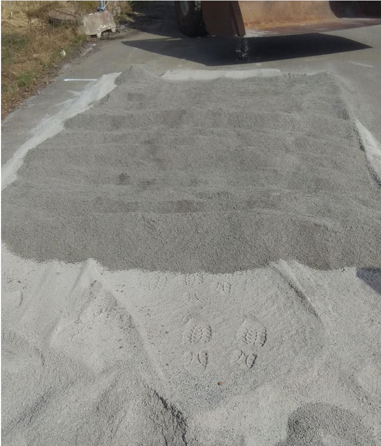
Figure 7. The first layer of 0/4 mm showing in light grey and the second layer in darker grey. It is evident that the material dried up rather quickly due to it being directly under the sun.
