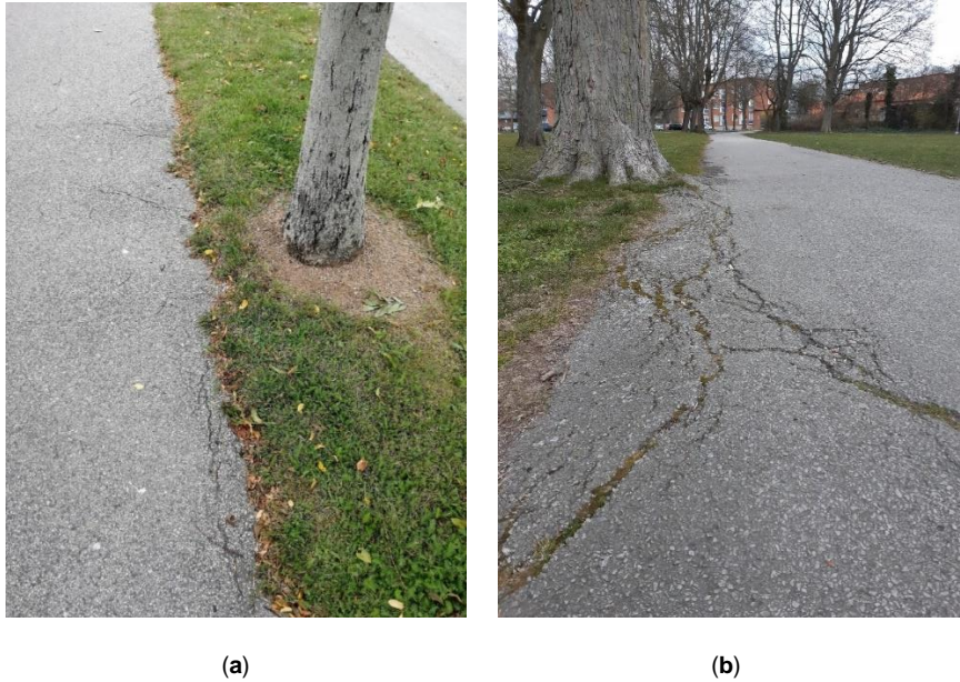
Figure 12. (a): Initial cracking of the asphalt concrete due to infiltration of roots from a tree that was placed too close to the edge of the cycle path. (b): Advanced cracking of the asphalt concrete from an old tree beside the cycle path. Grass intrusion of the cracks has occurred.
