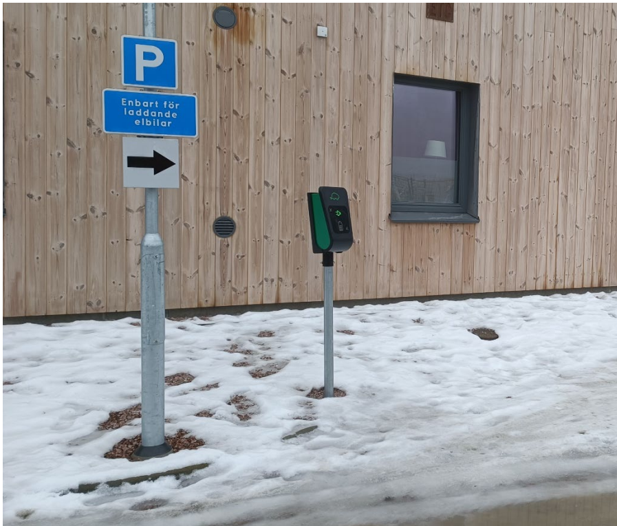
Picture. Parking space at the Västerås house - only for charging electric cars.
