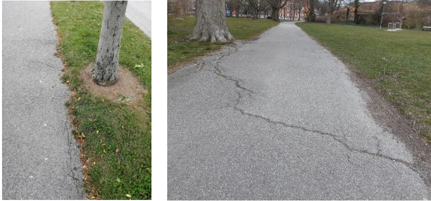
Figure 17. To the left: Initial cracking of the AC due to infiltration of roots from a tree that was placed too close to the edge of the cycle path. To the right: Diagonal crack that spans the whole width of the cycle path.
