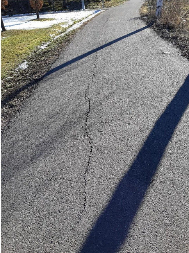
Figure 13. Frost heave, in the form of a longitudinal crack close to the centre line of the cycle path.
