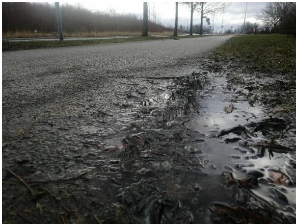
Figure 16. The lack of ditches and shoulders, in combination with deposited organic material—leaves in this case—results in standing water along the edge of the cycle path.
