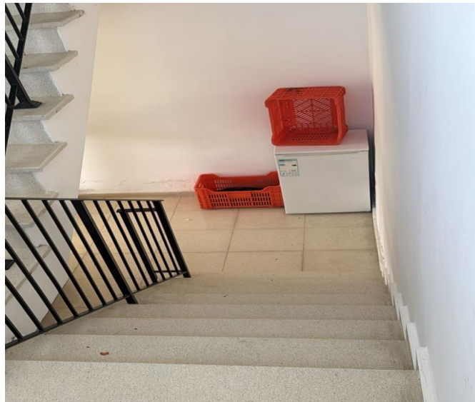
Figure 4.4. Objects on the emergency exit stairs.
