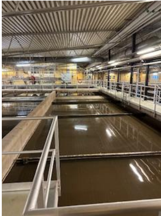
Figure 6: View of the clarifier units used to separate sludge from treated water—an important step in ensuring effluent quality.
